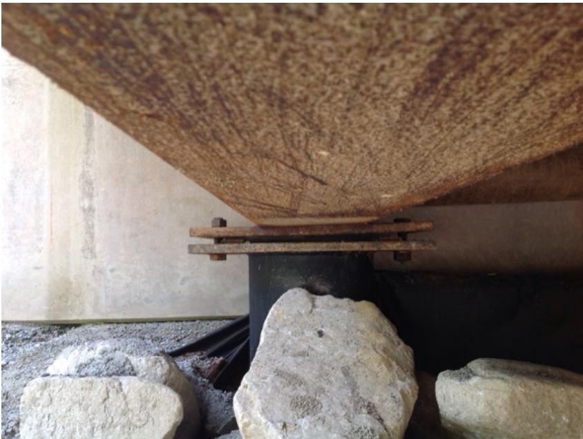
bearing plates slightly deformed on right bank and downstream left bank
