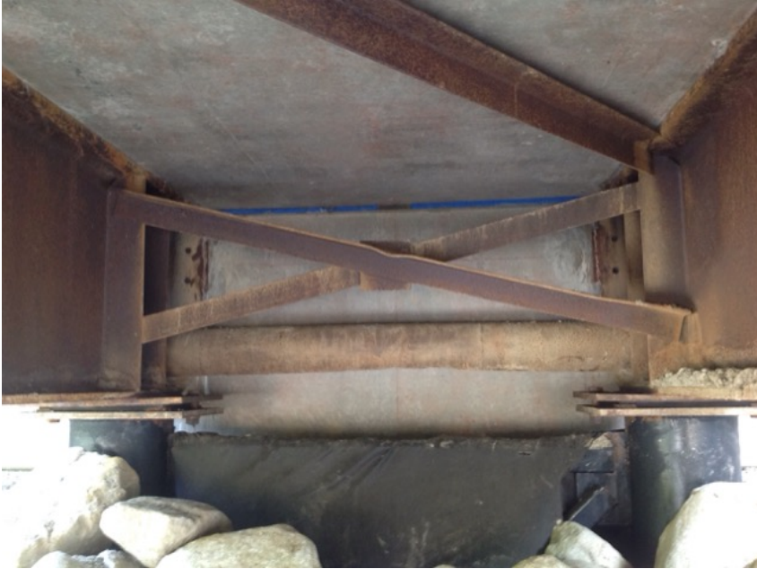
minor diaphragm damage
