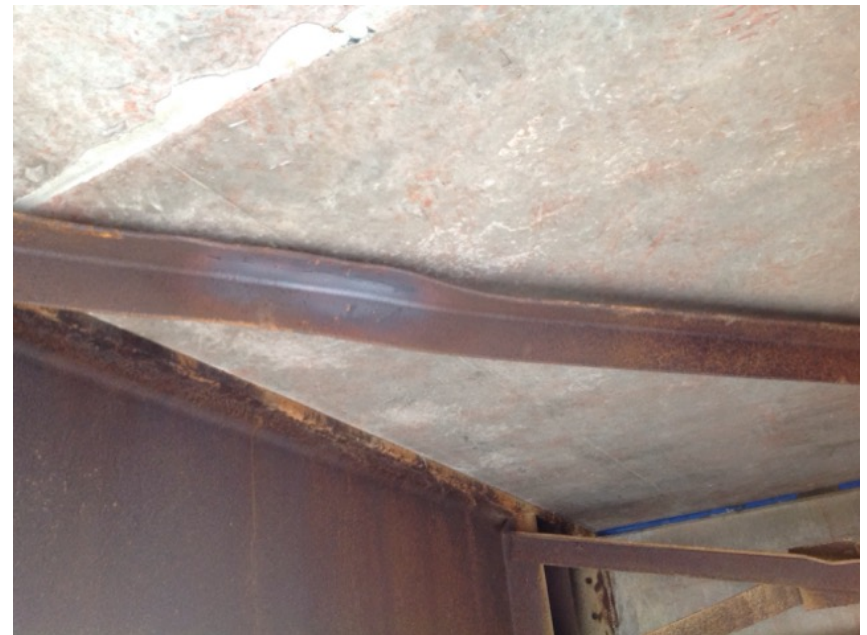
minor bracing damage
